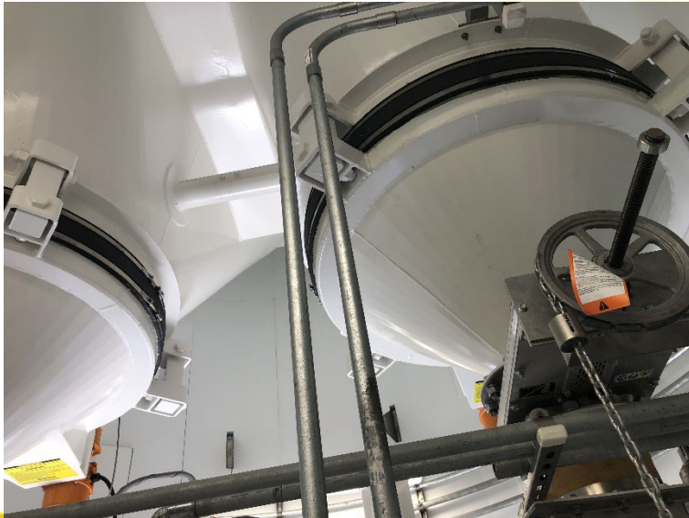
Inside the Lime Silo
